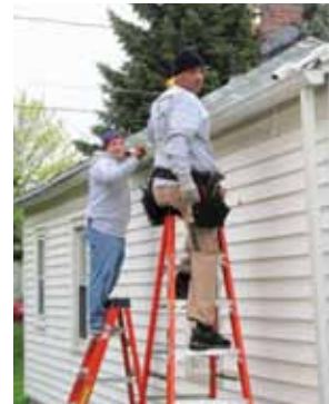
SDC Weatherization staff volunteer to put up new gutters on a home.
